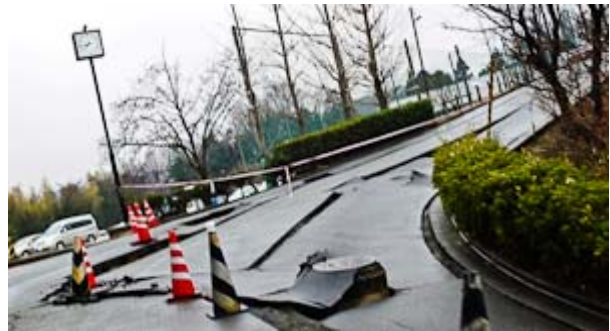
Damaged street - Iwaki
